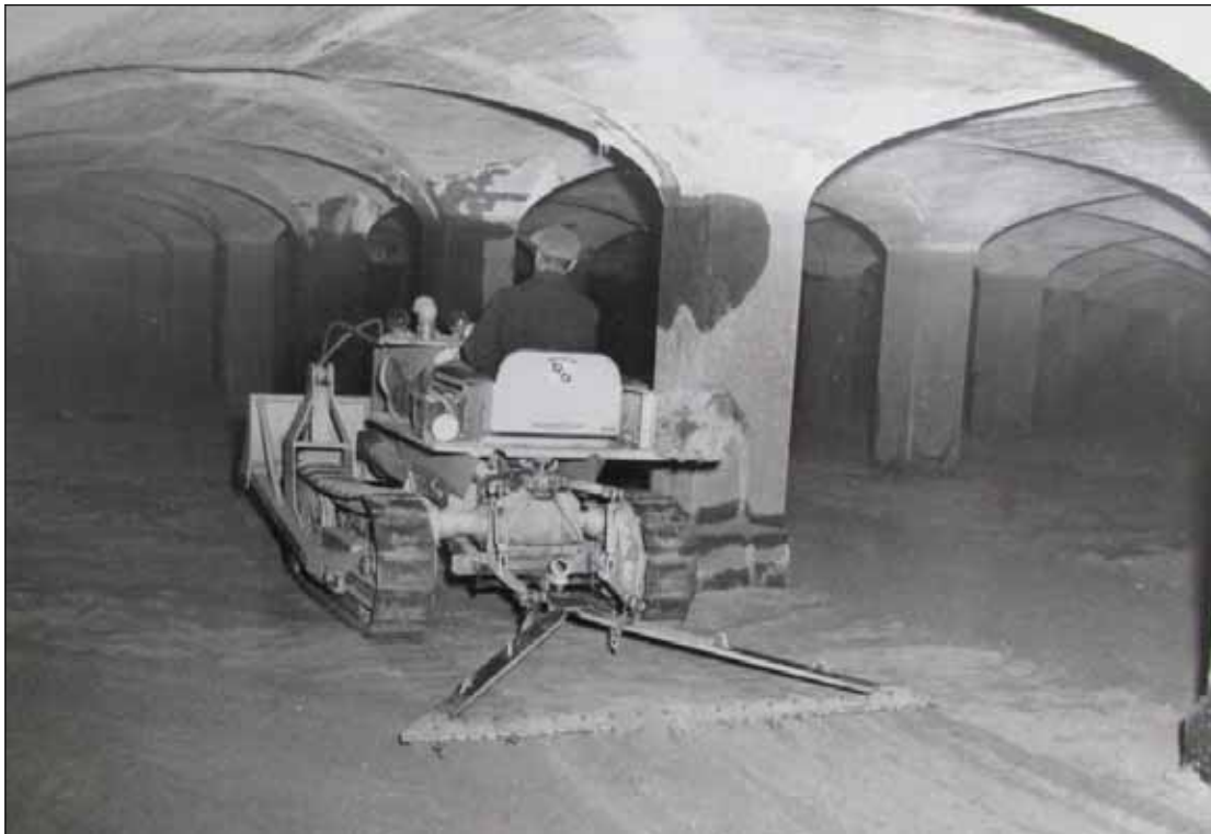
C-25: Tractor and filter rake pulverizing the filter sand surface and filter operation (c. 1944) Courtesy of the Archives of the Washington Aqueduct
