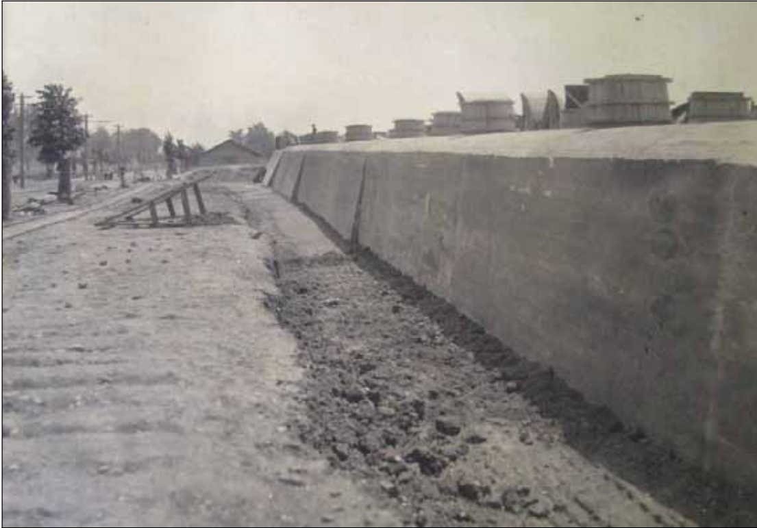
C-3: Concrete wall of filter beds (June 4, 1904) Courtesy of the Archives of the Washington Aqueduct
