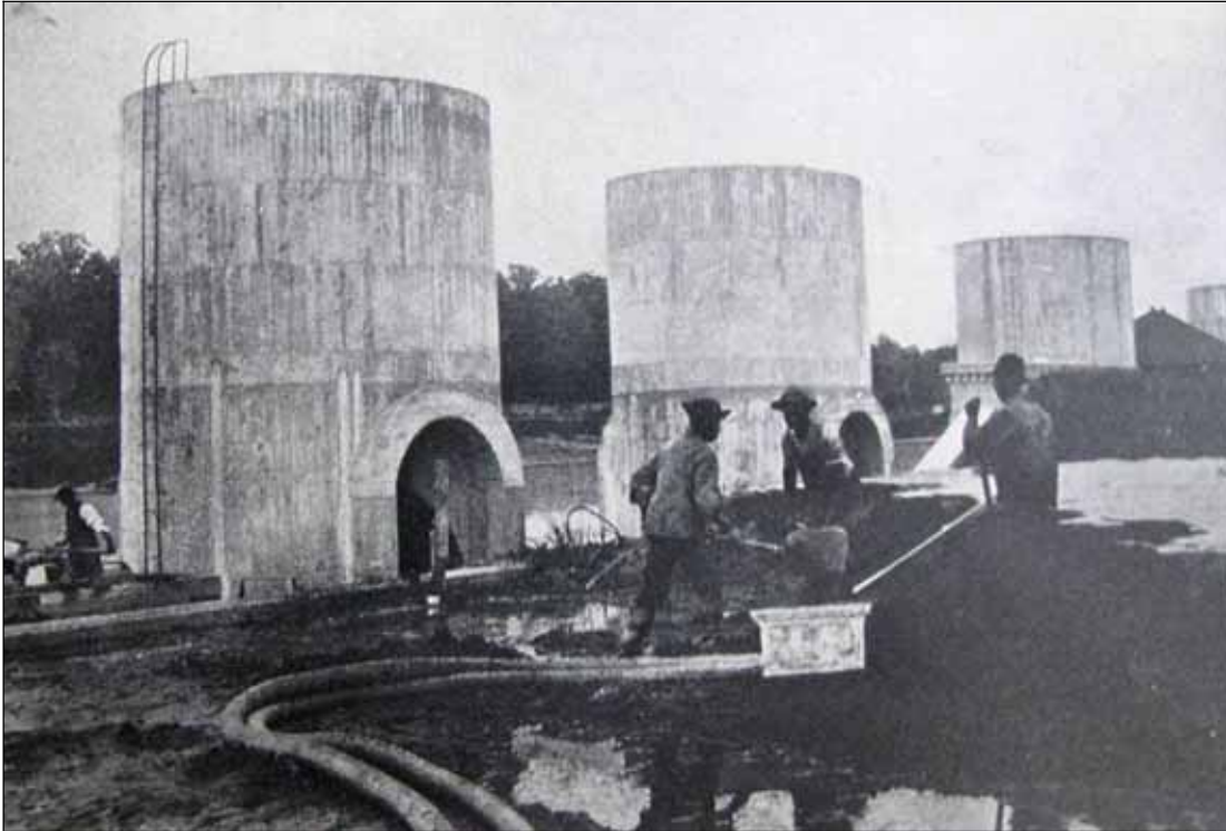
E-3: Movable ejector at work moving sand temporarily stored on top of filter (c. 1904) Purification of the Washington Water Supply (TD225.W3 A3 1909) (See Appendix A) Courtesy of the Historical Society of Washington, D.C.
