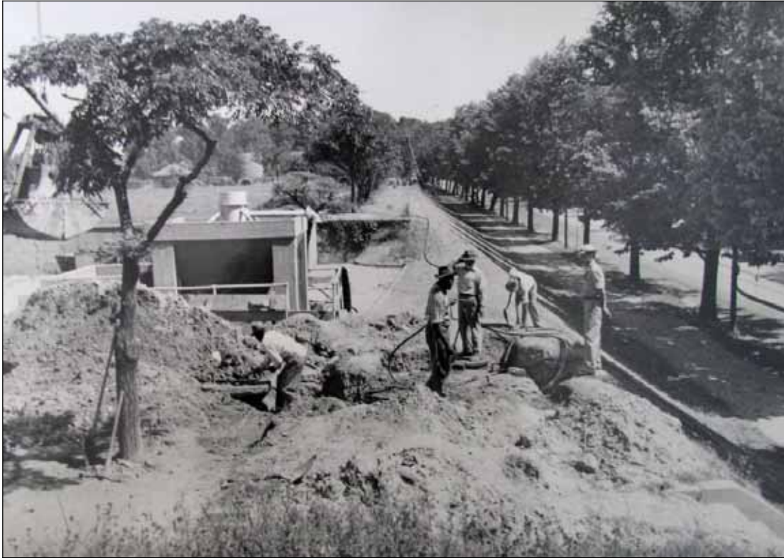
C-32: Construction of 36-in rising main loop, looking north on North Capitol Street from Court 2 (June 13, 1946) Courtesy of the Archives of the Washington Aqueduct
